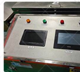
4. Control cabinet: Add a control box, neat and easy to clean
