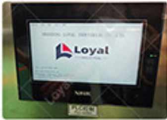
1. PLC control system
