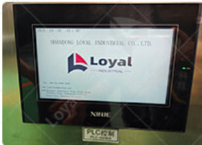
1. PLC control system
