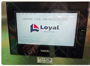
1. PLC control system
