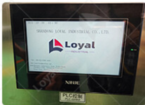
1. PLC control system
